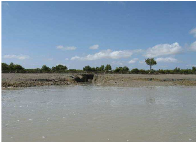
Figure 3-2: Example of near vertical drop off caused by severe bank scouring (Photo: ALS Water Science Group)
